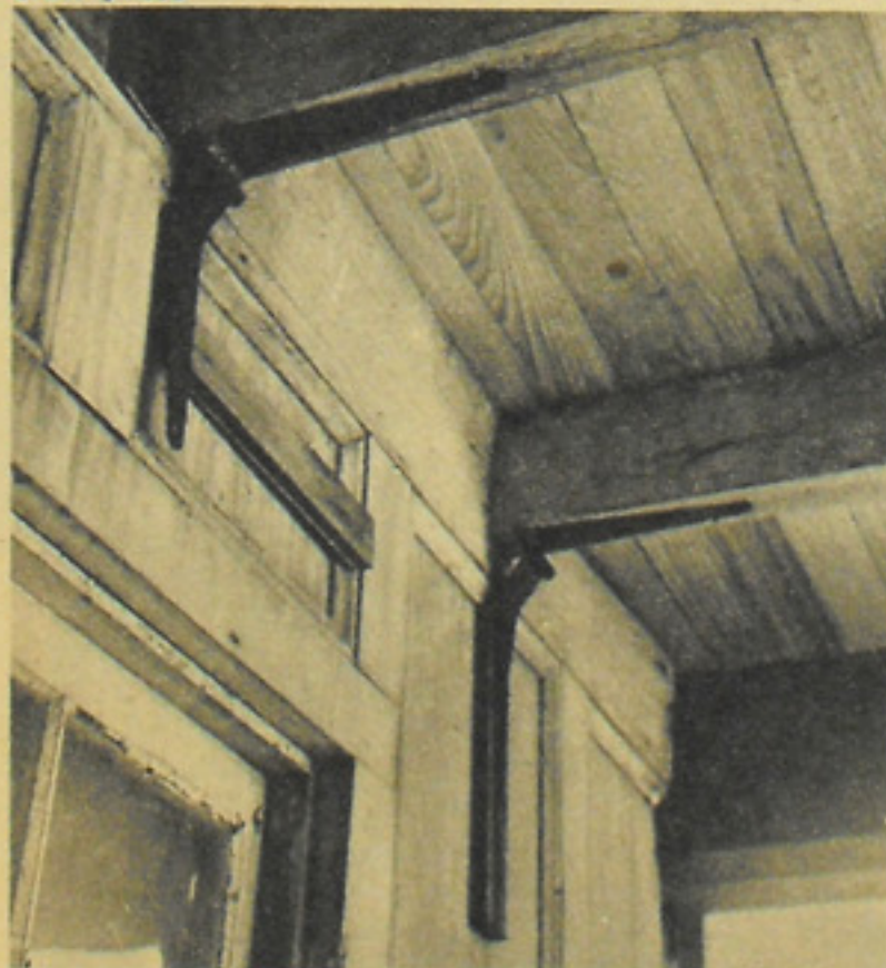
These king-size hinges were used to fold down ceiling of porch before the move. The porch floor was removed, later replaced
